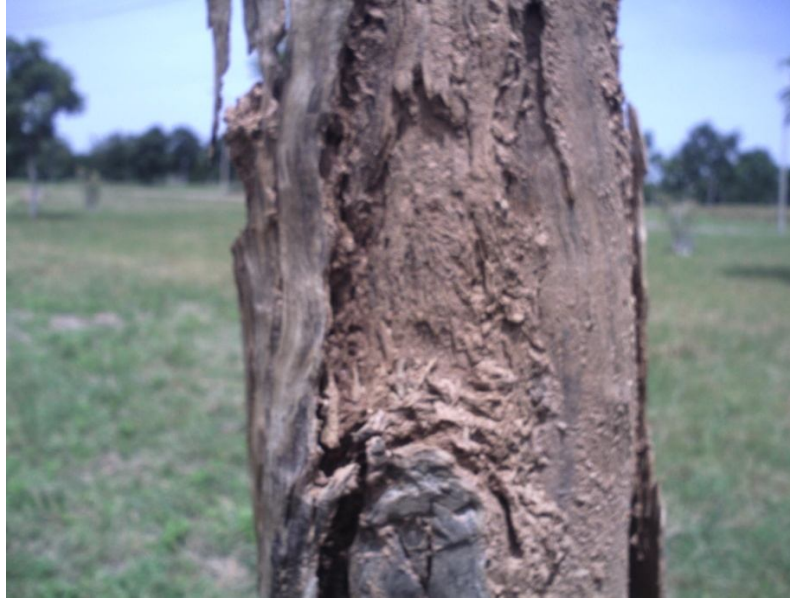
PLATE 5. ELECTRIC POLE FROM Eucalyptus camaldulensis DEHNH. ATTACKED AND DESTROYED BY TERMITES Odontotermes sp.
