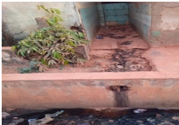
Plate 1: Open Defecation close to a Drainage in Tudun Wada, Zaria LGA Source: Fieldwork (2025)
